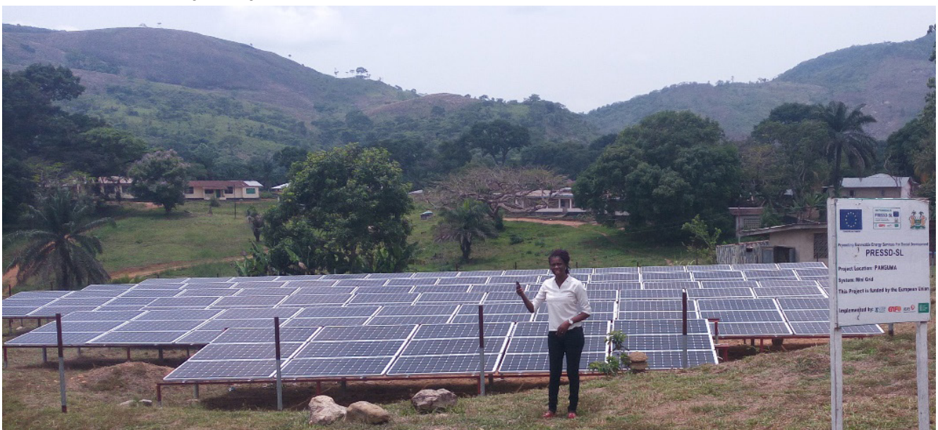
Solar Pannels at Panguma
