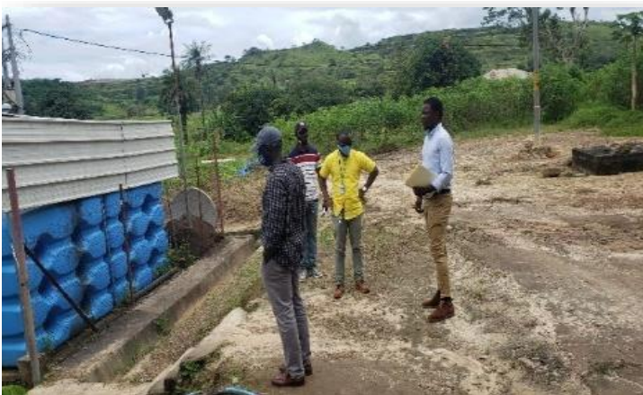
Dilapidated Ultrafiltration Membrane System-
